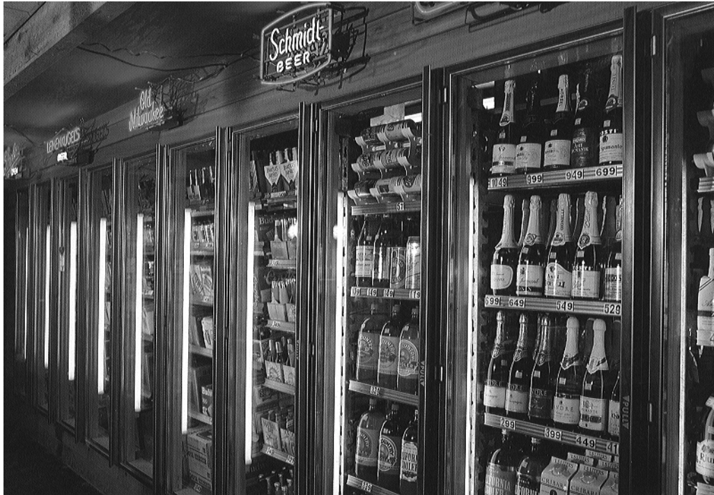
Figure 4-36: A Walk-in Cooler with Merchandising Doors
